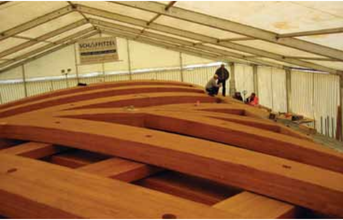
To prepare for final assembly, workers placed a large tent over the shells and heated it. After this, the bonding of the threaded rods using the prepared holes could take place.
