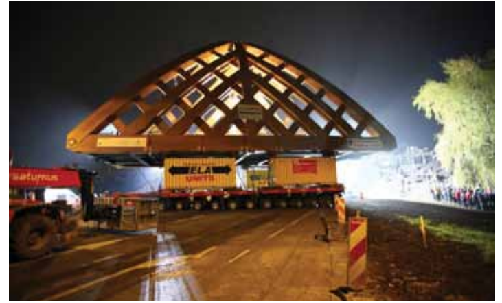
Two self-propelled modular transporter (SPMT) vehicles were used to move the 400-ton bridge 2,624 feet, 8 inches from the assemble area to the final location.
